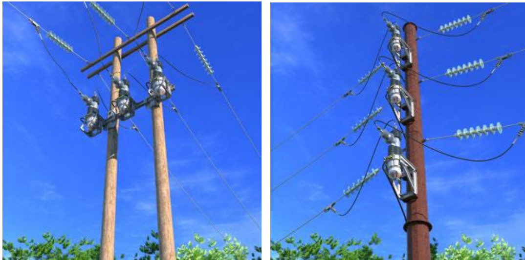
High-Voltage (72 kV) Sub-transmission Pole Top Recloser
